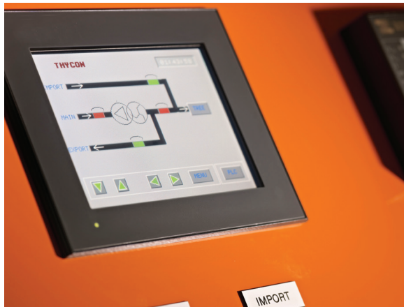
Multi Circuit Monitor Display
